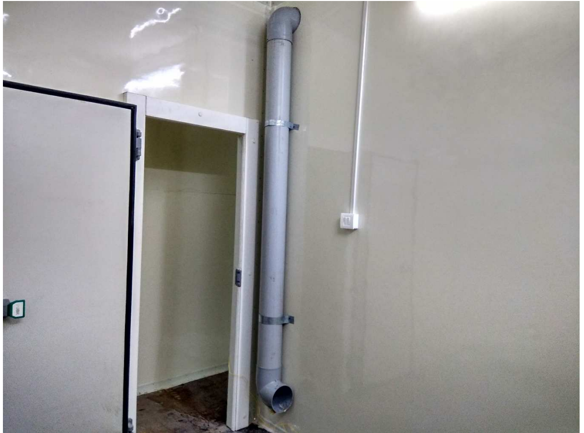
Exit pipe to solar collector for air recirculation
