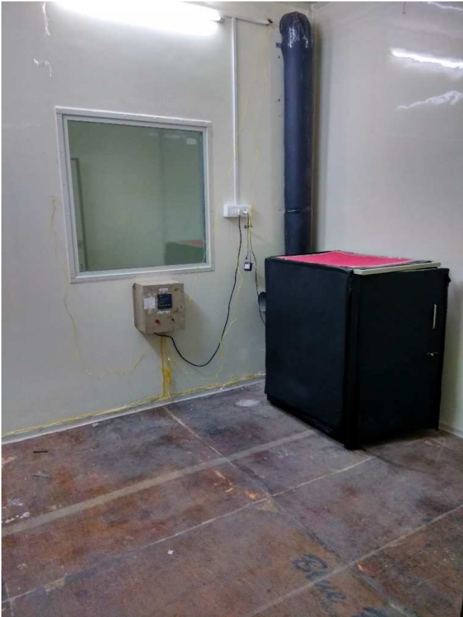
Heat exchanger set up in the room
